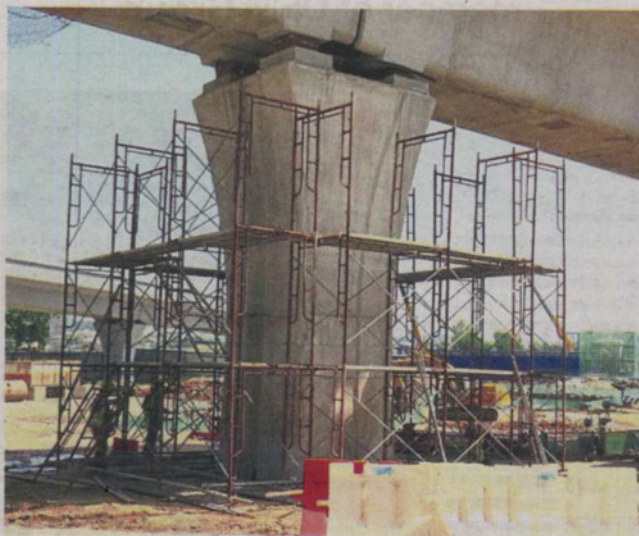
MRT job: The Klang Valley Mass Rapid Transit line is one of the two main projects undertaken by Sunway Construction Group.
